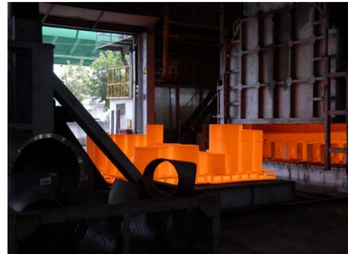
Solution Heat Treatment Furnace
