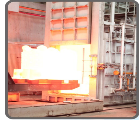
HEAT TREATMENT FURNACE
